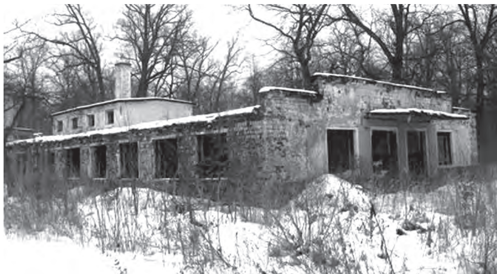
An abandoned building (future site of the pig farm) at the Nazareth Rehabilitation Center's facilities.
