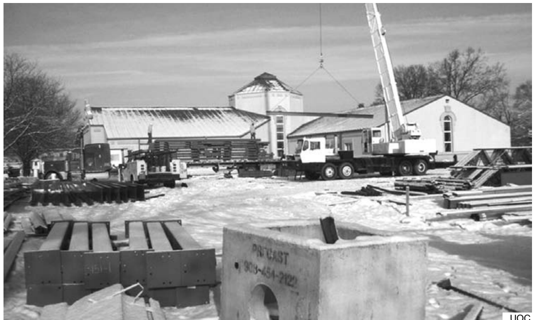
A view of the construction site of the Patriarch Mstyslav I Ukrainian Orthodox Museum.
