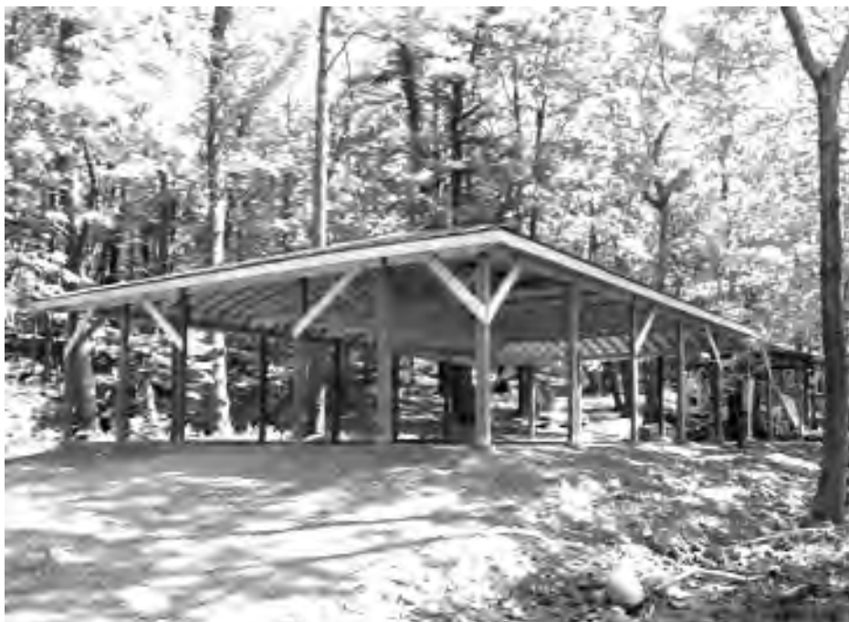
The dining hall for older boys under construction at Plast's Vovcha Tropa campground in early 2006.
