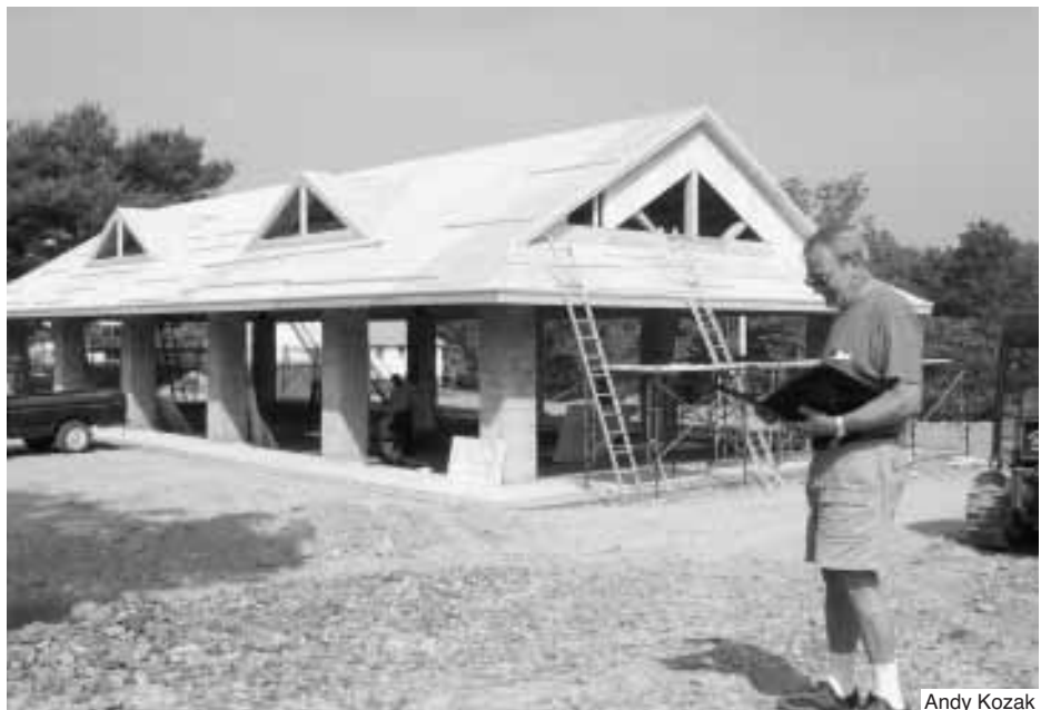
Petro Bokalo inspects the pavilion under construction at Plast's Vovcha Tropa campground.
