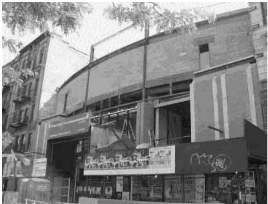
The exterior of The Ukrainian Museum's new building in New York City.
