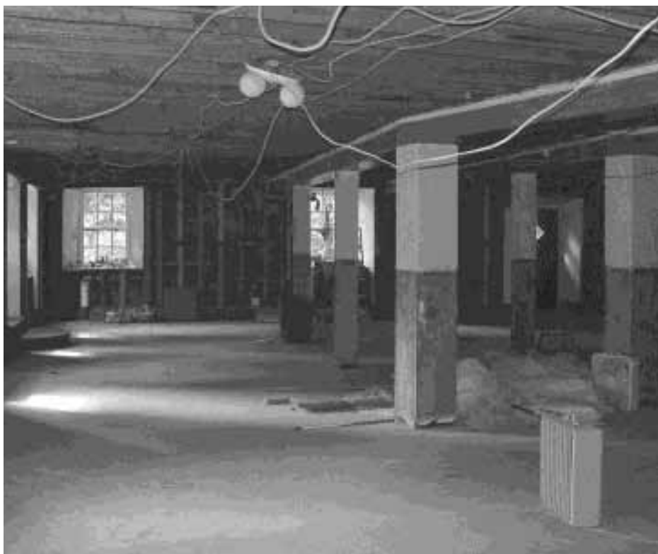
The dining room in the Main House as it looked when it was gutted.
