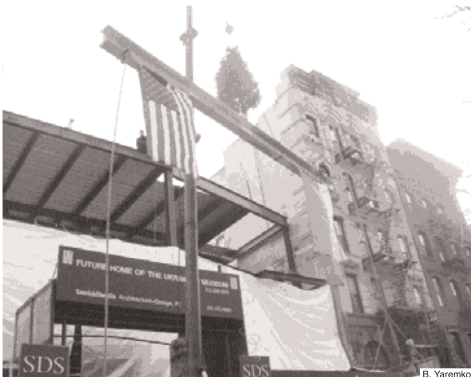
The steel beam rises to the top of the infrastructure of the museum's future home.
