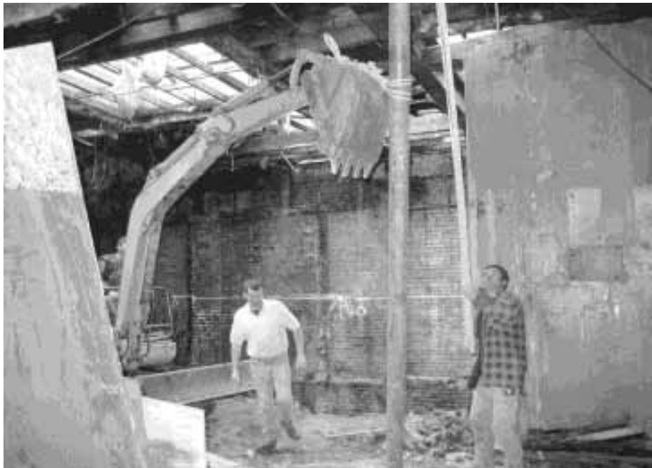
Interior view of existing structure where "underpinning" is in progress in the construction process of a new Ukrainian Museum building.
