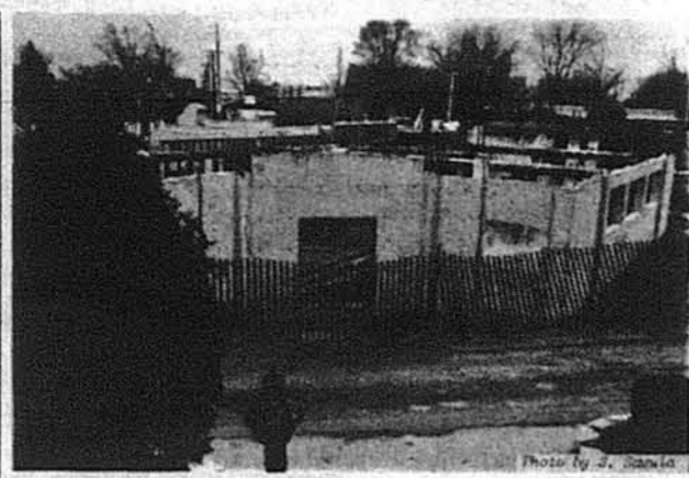
Progress on the construction of St. Joseph's Ukrainian Catholic Church in Chicago as it looked at the close of last year.
