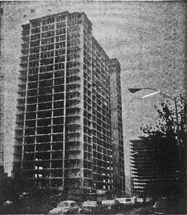
1,000 above shows the 23-story Paulus Hook Towers in Jersey City, now under construction. In the background is the steel frame of the UNA skyscraper, scheduled for completion early next year.
